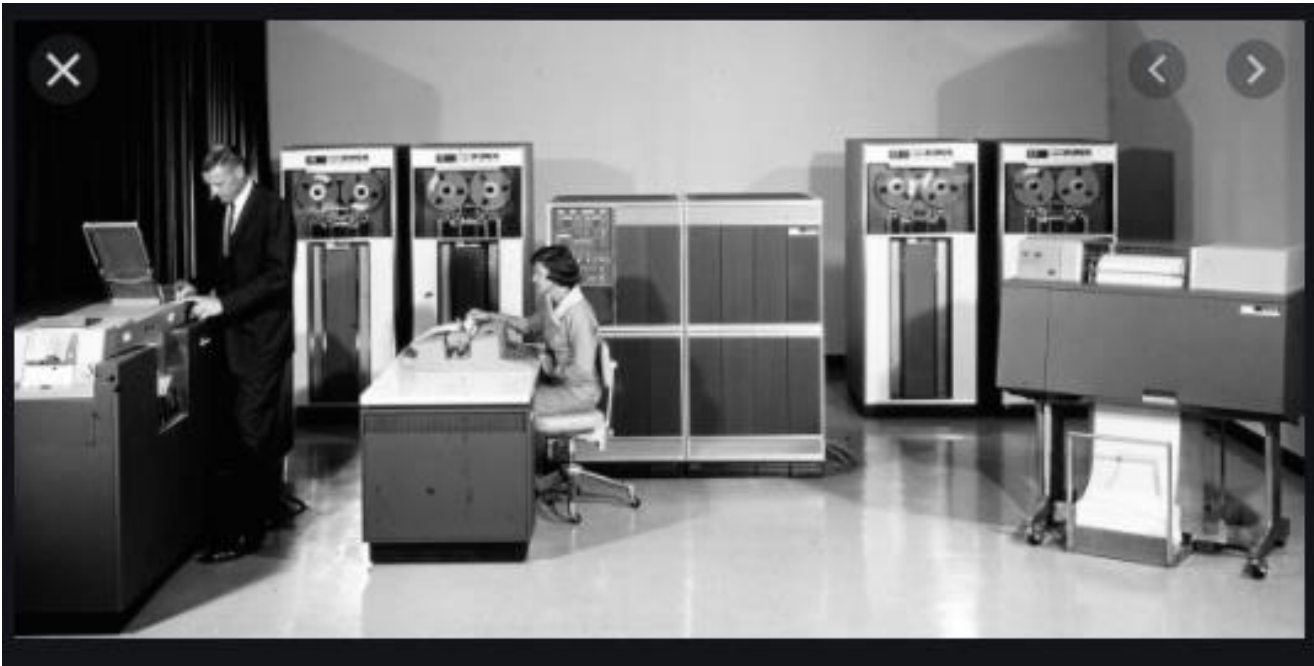
This is most of an IBM 360 mainframe installation! The big box in the middle was about 1/12 th of the size of the previous computers – the result of shifting from tubes to solid-state circuits. The “admin” monitored all programs and output – programs ran one at a time!
